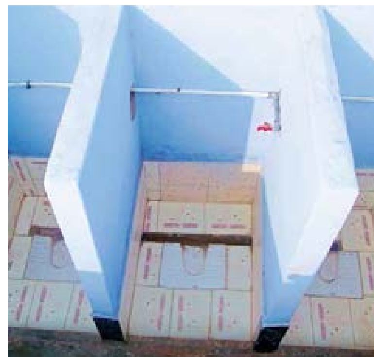
Running water inside the urinals ensures that the structure is well maintained
